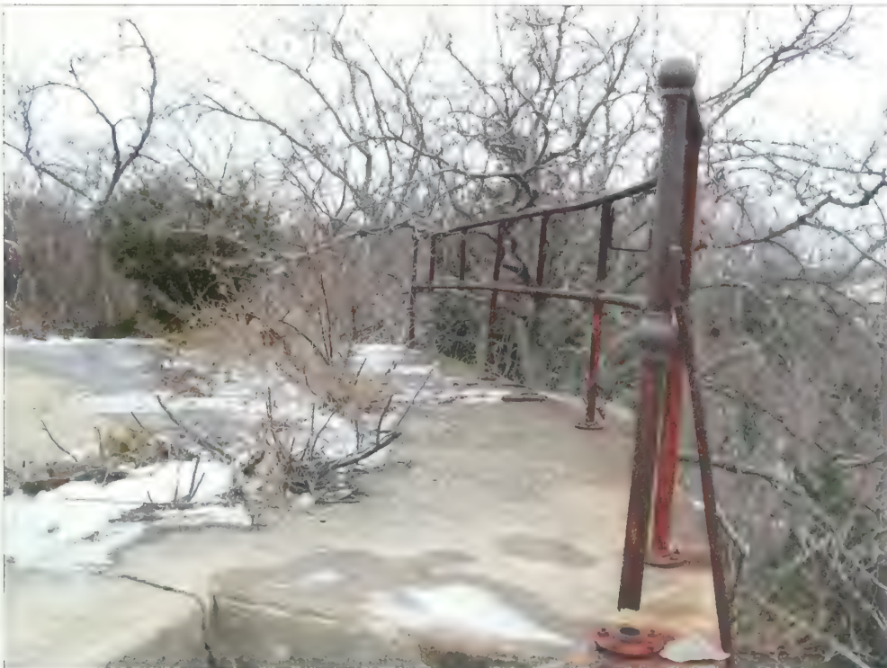
Figure 5.40. View of historic guardrail south of emplacement #1, Battery Peck. Severely deteriorated railing components, such as the vertical post in the foreground, should be removed and replaced with new components that match the original as close as possible. Final painting or a color-galvanized coating should match the historic railing paint finish (Olmsted Center, January 2009).
